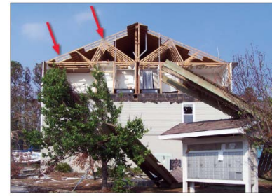
(c) Gable end and side wall failure in Andrew (FEMA 1992)
