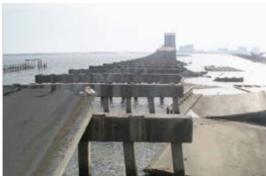
Fig. 3 Span Unseating of US-90 Biloxi-Ocean Springs Bridge
