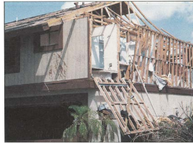
(b) Gable end wall and roof edge sheathing (arrows) failure in Katrina (FEMA 2006)
